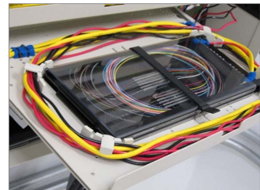
Cable Head End (Source: City of Bellevue)
