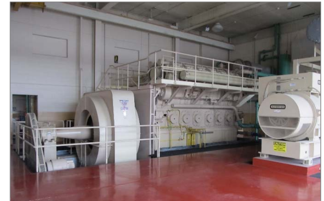
Bellevue Electrical Power Plant (Source: City of Bellevue)
