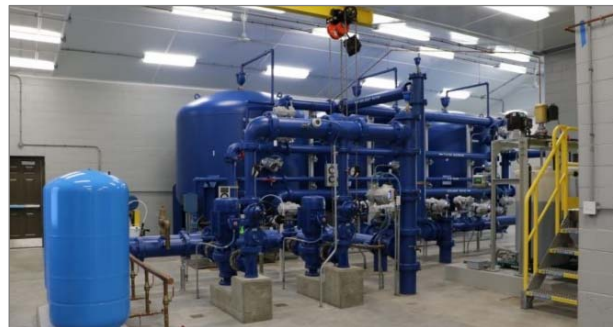
Bellevue Water Radium Treatment Plant (Source: City of Bellevue)
